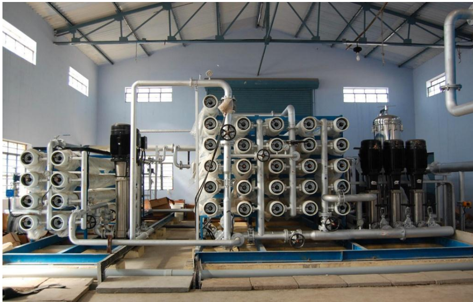
The reverse osmosis system is an important feature in our zero-liquid discharge plant in Perundurai, India.
