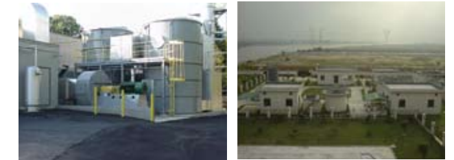
Oxidizer for Air Pollution Abatement—A&E Plant, NC, USA
