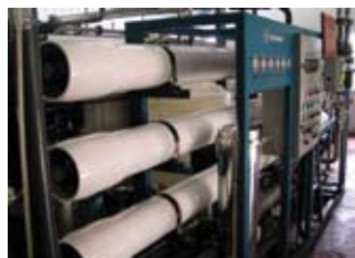
Wastewater Purification and Reuse System—Reverse Osmosis at A&E Sri Lanka
