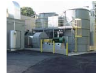
Oxidizer for Air Pollution Abatement—A&E Plant, NC, USA
