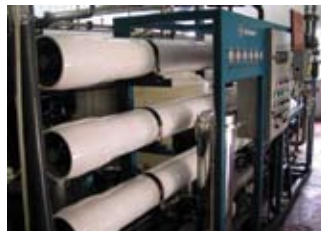
Wastewater Purification and Reuse System—Reverse Osmosis at A&E Sri Lanka
