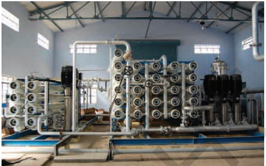
Reverse osmosis is a key element in the zero liquid discharge plant at Perundurai in India.
